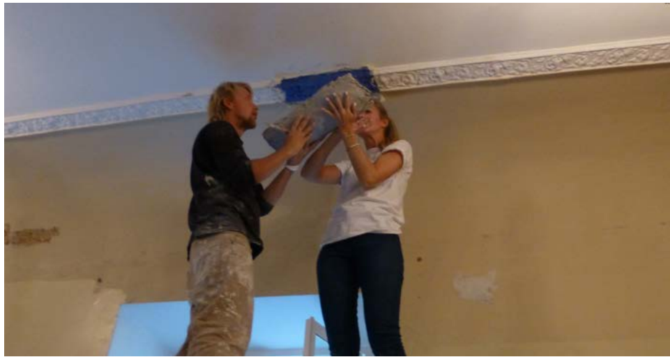
Figure 2.22. The moulds were taken down the next day. Photograph by Kirsti Horn.
