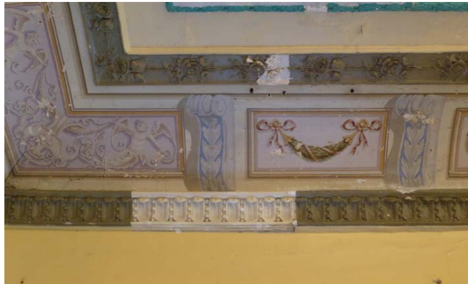
Figure 1.2. The cornice of the ballroom in Voltveti manor consists of three lines of decorative plasterwork and trompe l'oeil painting with consoles, putti and garlands in between. Photograph by Kirsti Horn.
