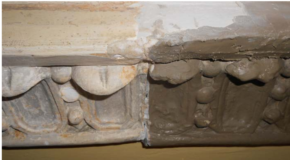
Figure 2.2. The removal of paint revealed bad joints between the precast sections. Photograph by Kristiina Ribelus.
